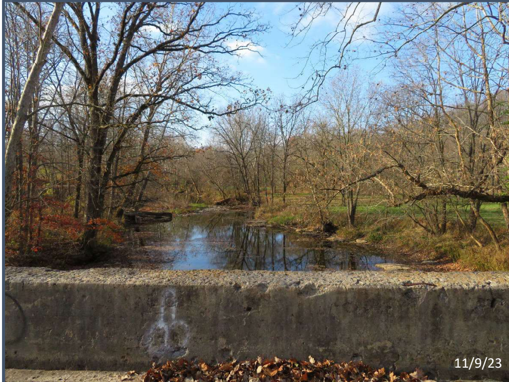
4) Looking west (downstream) at Leatherwood Creek from west side of the center of bridge 172
