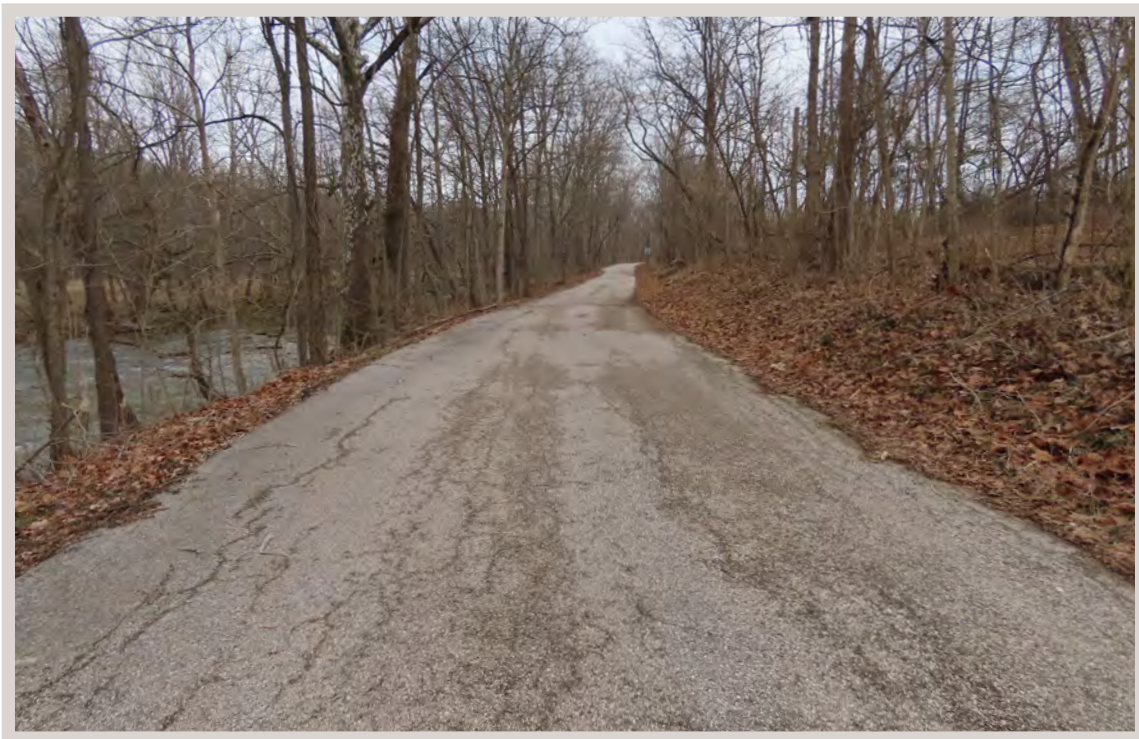
Photo 10: Looking northeast along Cement Plant Road from the farthest potential eastern terminus of the project area.
