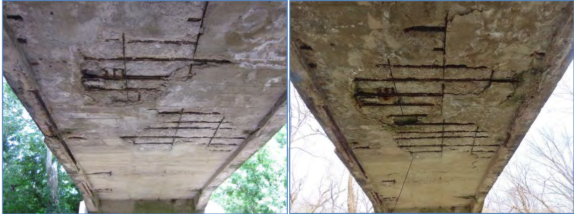
Figure 1. Underside of Span B in 2014 (left) and 2022 (right)
